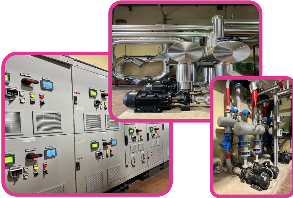
Photo of the district heating system at the Rozzano Data Center
